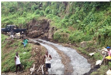
Making a new road to Megamone after the cyclone and subsequent rain washed away all access! Making use of bags of cement that would have otherwise been ruined
